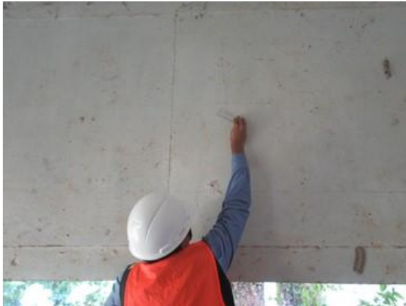
Foto 16: Viga transversina 4 – Face – Fissura vertical.
